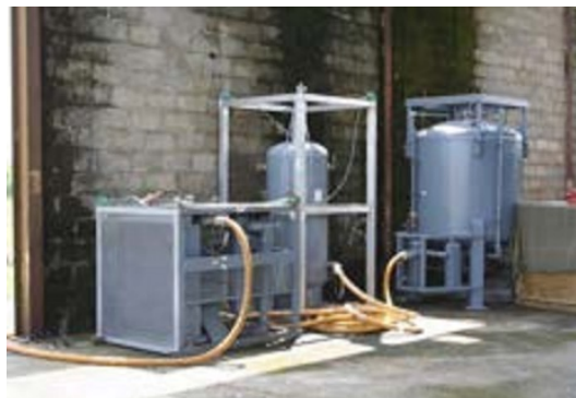
4# Blasting & Painting Equipment
